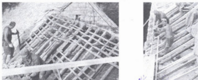
Fig. 7 – New rafters are added to the olds, new eave is reinforced by concrete
